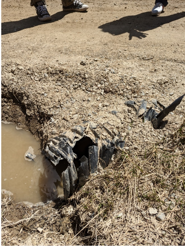
Figure 4. Downstream side of existing cross culvert at Sherwood Lane and Starlit Lane. Poor drainage from culvert was observed.
