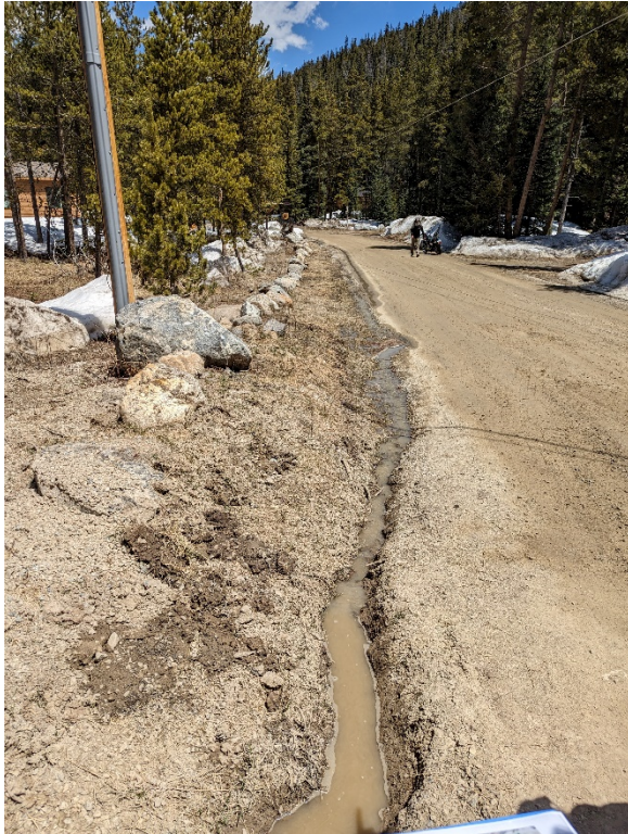
Figure 3. Downstream side of existing cross culvert at Sherwood Lane and Starlit Lane. Looking east along Sherwood Lane.
