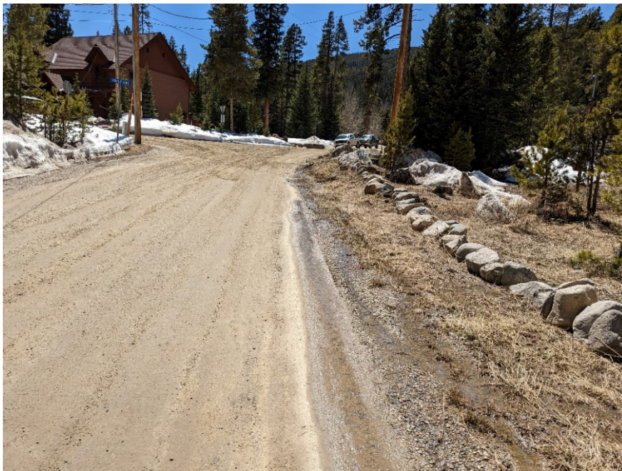
Figure 5. Sherwood Lane. Looking west at the intersection with Sherwood Lane and Starlit Lane. Drainage along the existing roadway corridor was observed.
