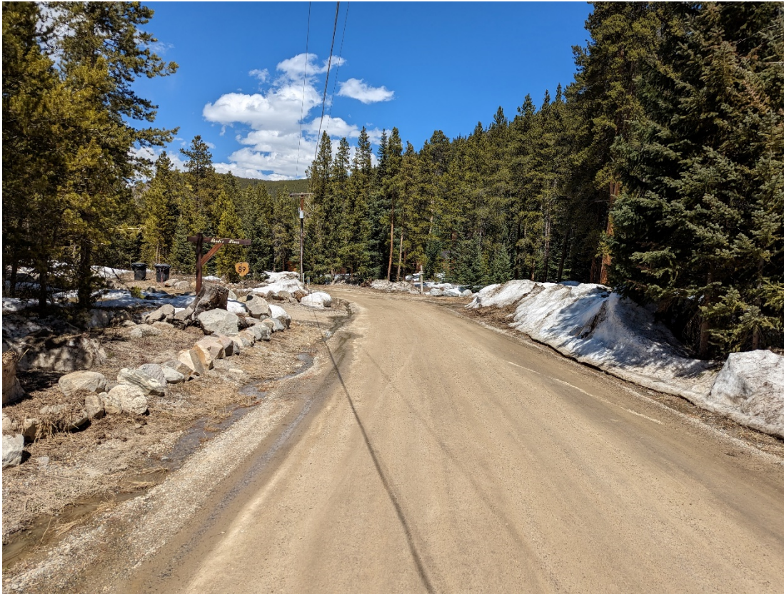
Figure 6. Sherwood Lane. Looking east. Drainage along the existing roadway corridor was observed.
